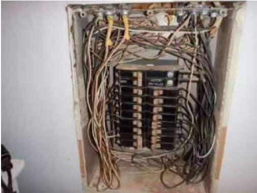
Photo 11-1 Cutler & Hammer Brand Panel 100 Amp Service
