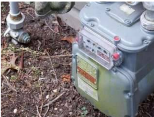
Photo X-11 Gas Meter outside
